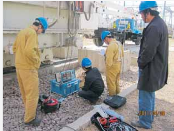
500kV Tranformer Bushing CT
